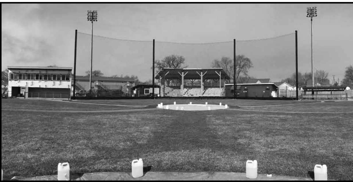
The view of the new grandstand and press box over the first base dugout as construction nears completion just in time for the Blue Devils' 2016 home opener on Tuesday, March 22 against Fort Calhoun.
